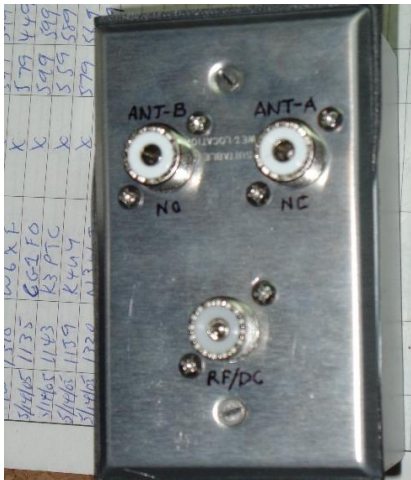
Photo C: Outside Unit – External View
