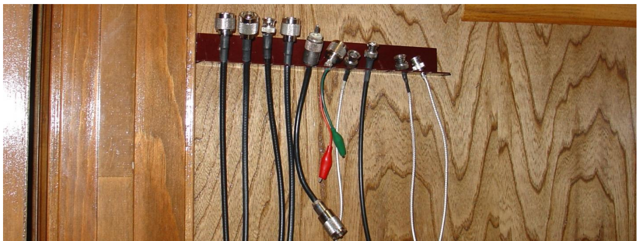
Photo B: Cable hanger in place on wall
