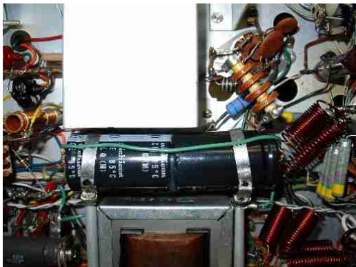
HV Capacitor and Grid Resistor
