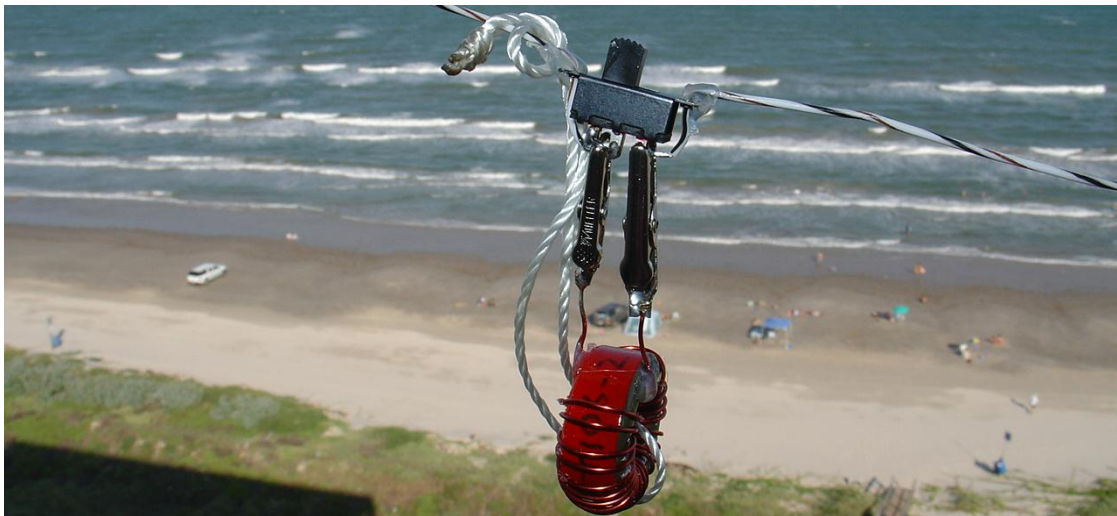
Figure 8: One 30 meter coil clipped across one 10 meter open switch
