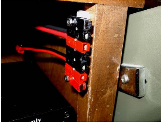
Assembly mounted in place
